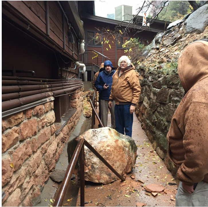
Photo P08. A large fallen boulder near Zion Lodge. Document consequences to structures and occupied areas as well as the rock source. People provide context, not a surveyed measurement scale. NPS / M. Reed. Source; Public domain (NPS credit) .
